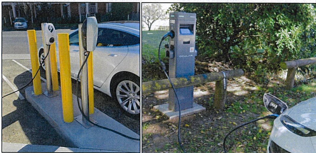
Bathurst Regional Council – Level 2 destination charging (‘wall mount’ left, dual port right)
